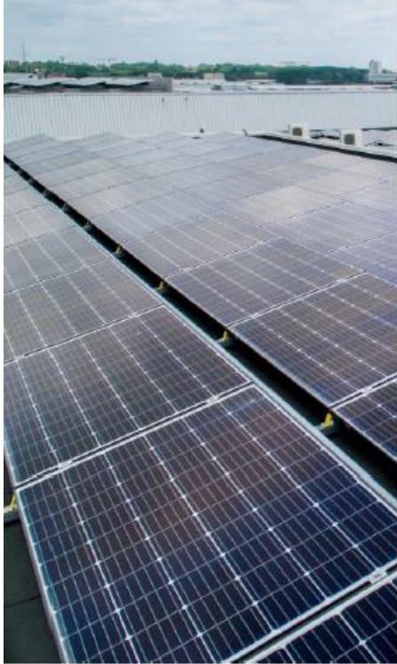
Solar panels above the workshops
